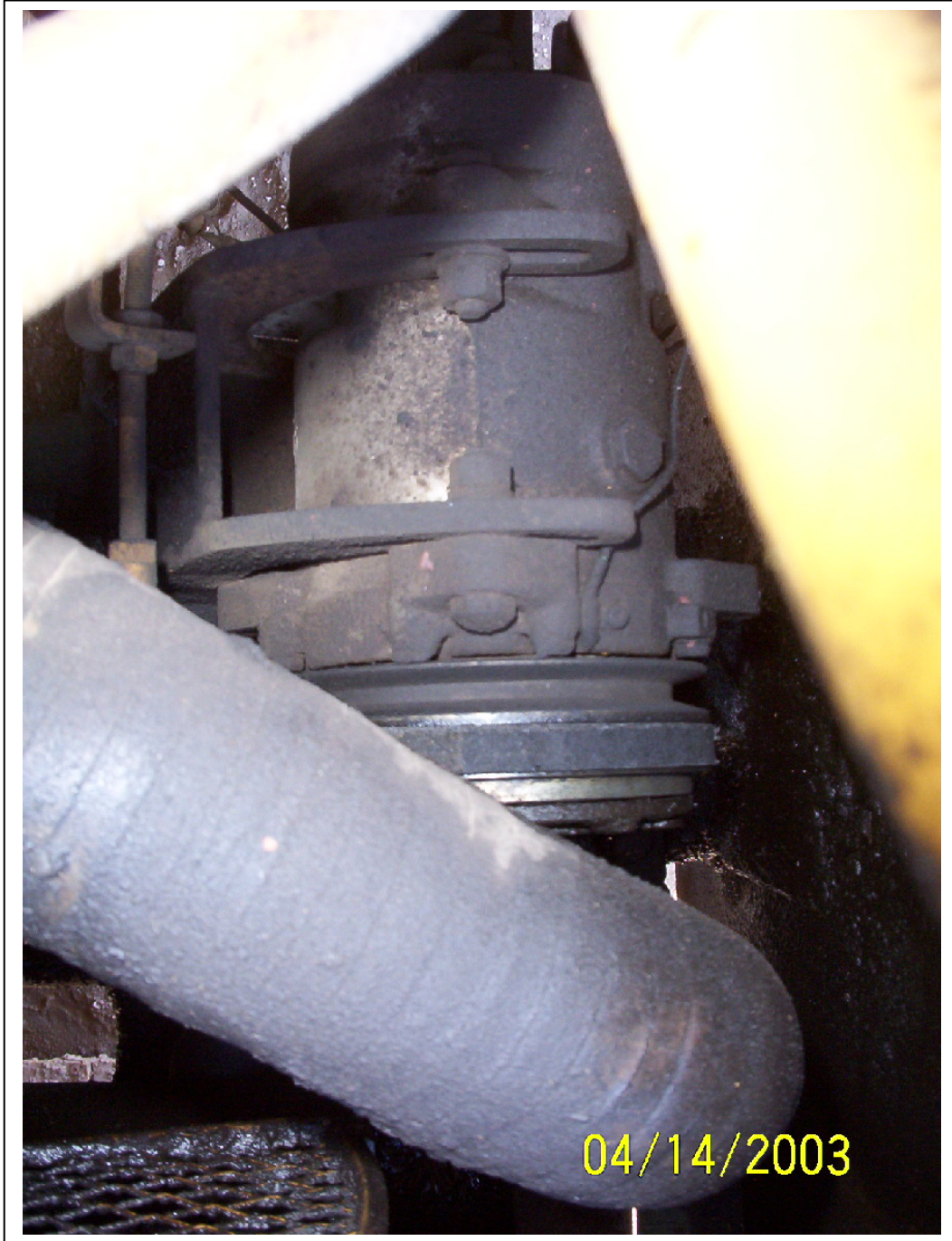
Top view of compressor in place
