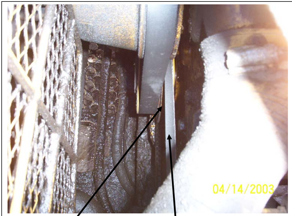
Open pulley for compressor belt
